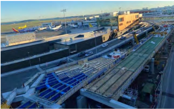
L1332-C4 Terminal B-C Main Roadways Logan Int'l. Airport Massachusetts Port Authority - Stantec
